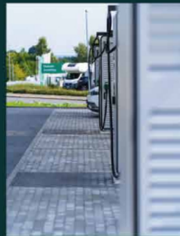
6 Electric Car Charging
